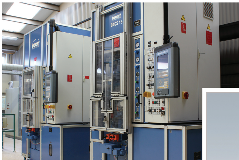
Dorst Dacs 30 and Dorst Dacs 15 installed in their new home
