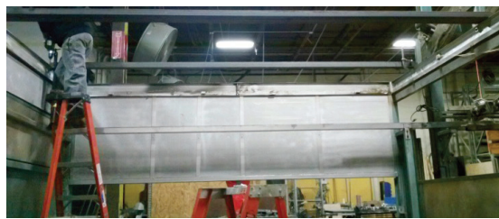
A view of the new IR platen being fitted and the new top and bottom quartz platens in place
