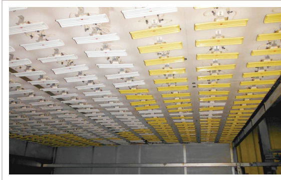
A view of the old oven using a competitors components and no reflectors, that was replaced with a full system build from Ceramicx and Weco
